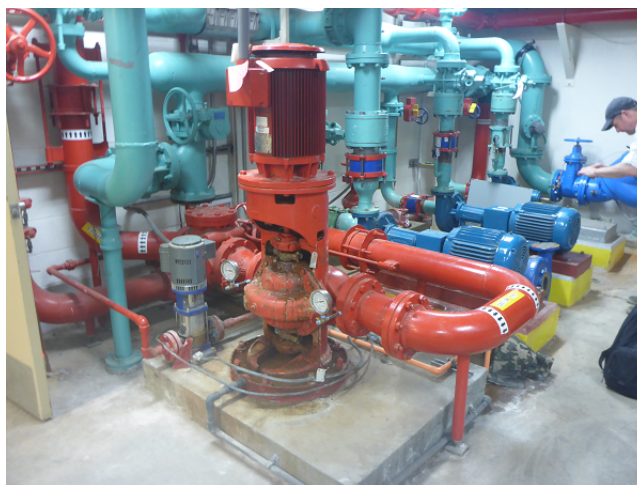
Existing Fire and Utility Water Pumps
