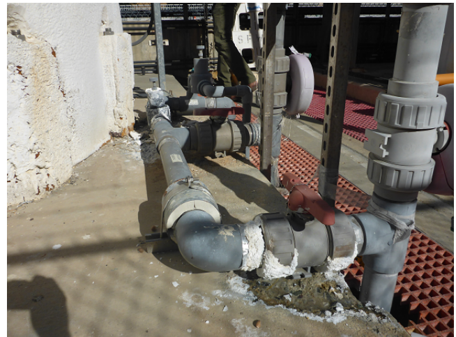
Concrete Damage at Caustic Soda Line
