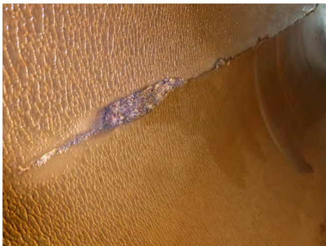
Typical Lining Failure
