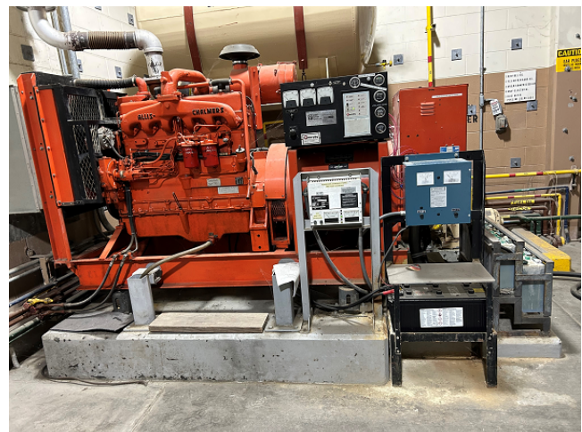
Existing Diesel Emergency Generator being Replaced with New Propane Generator to Backup SAPS Facility
