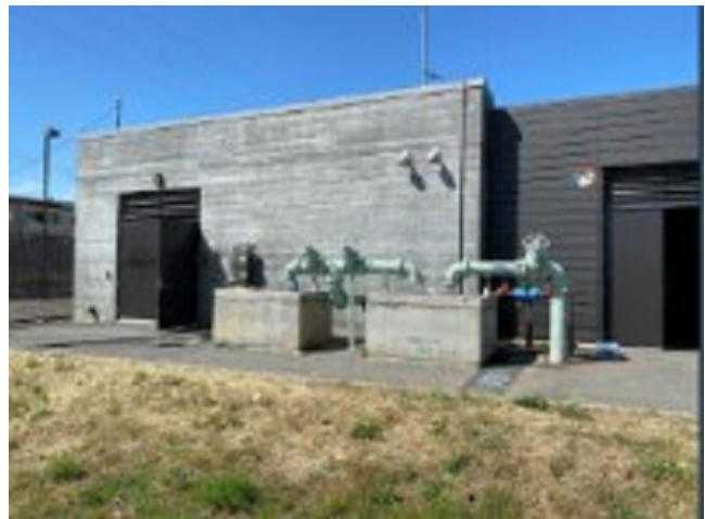
Typical Well Station
