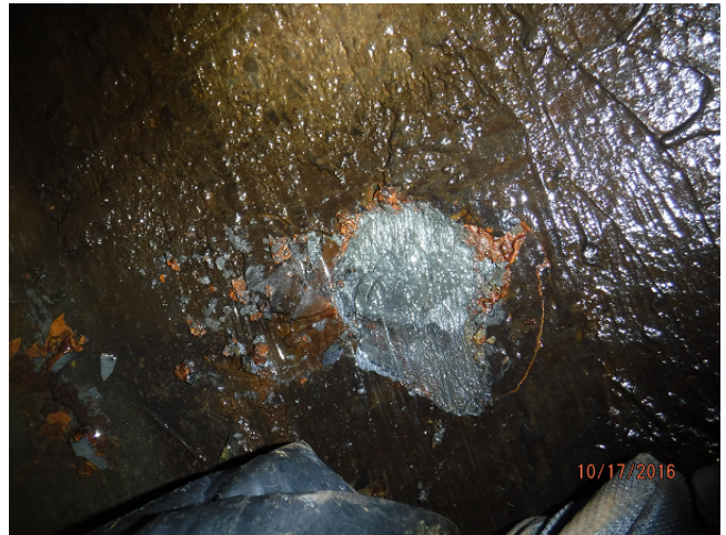
Typical Lining Failure
