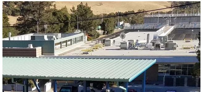
Administration Building Roof and HVAC system
