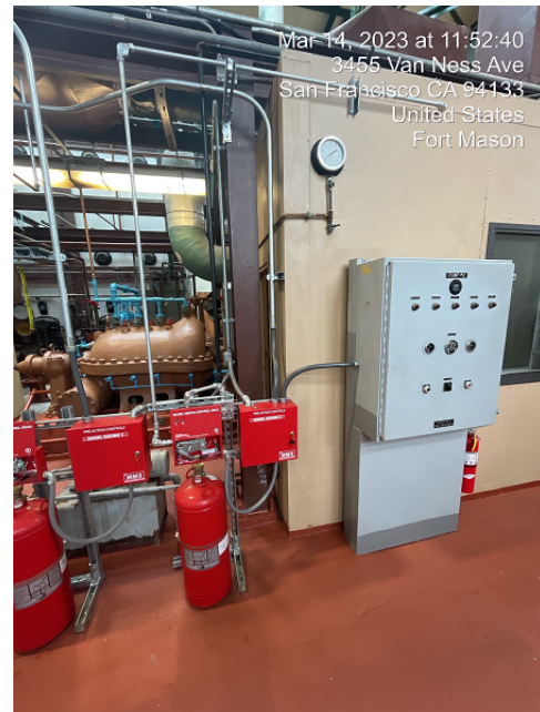
EFWS Pump Station No. 2
