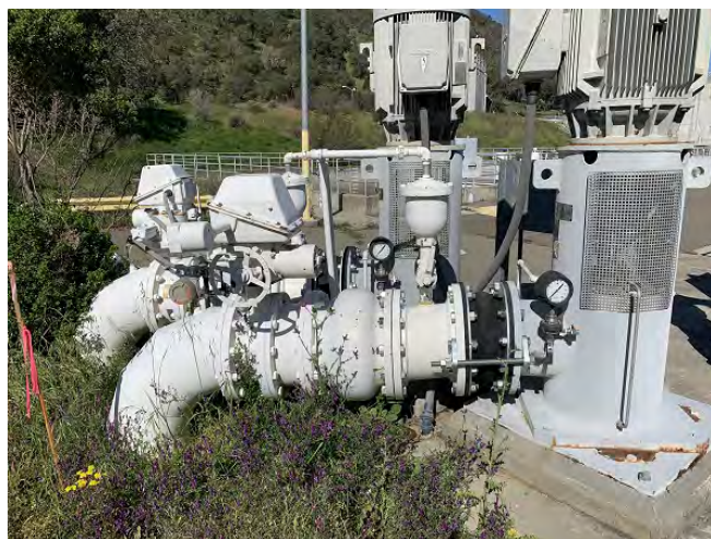
Existing Washwater Recovery Pumps
