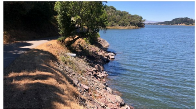
In-going Road-1 (IGR-1) along the west side of San Andreas Reservoir facing north along In-going Service Road.
