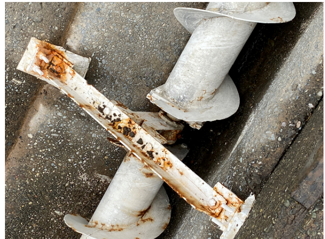
Existing Sedimentation Basin Cross Collector Corrosion
