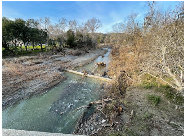
January Storms Further Expose Town of Sunol Pipeline and Tree Debris within the Creek
