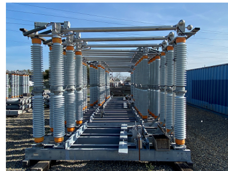
Top: Example of 35% Design Package Drawing Bottom: High Voltage Disconnect Switches (WSR Phase II)
