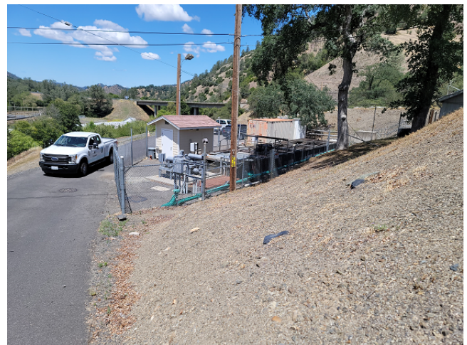
Existing Moccasin Wastewater Treatment Plant
