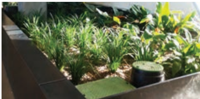
2nd stage of wetland treatment in building's interior (image courtesy of Denver Water)
