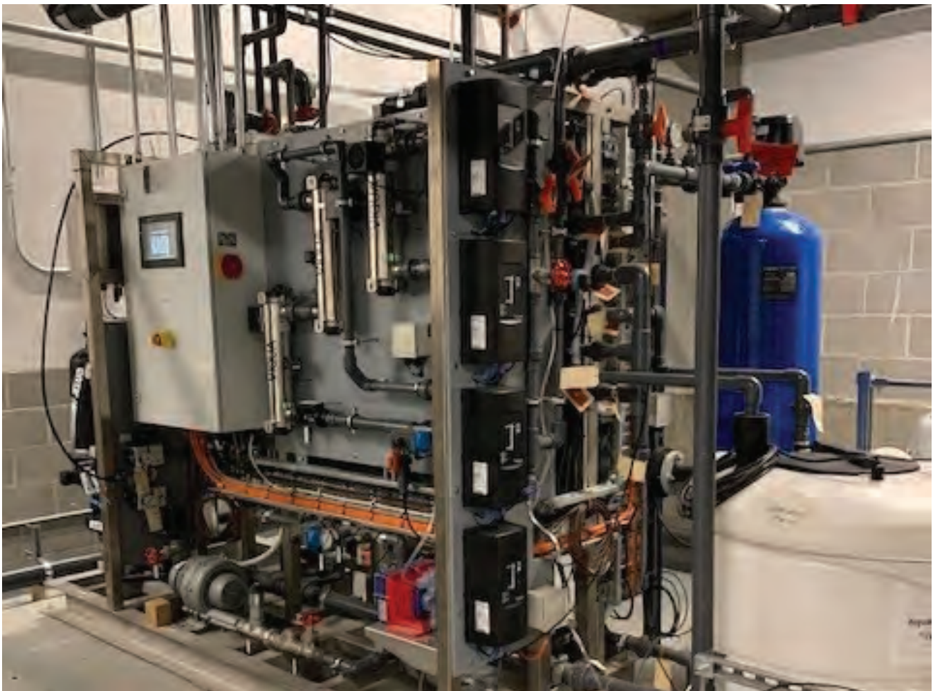
Onsite reuse system treatment skid at 49 South Van Ness (image courtesy of Aquacell)
