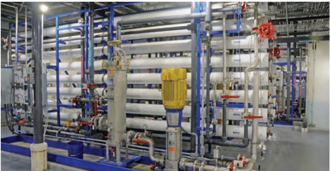
The onsite reuse system's mechanical room (image courtesy of Sustainable Water)
