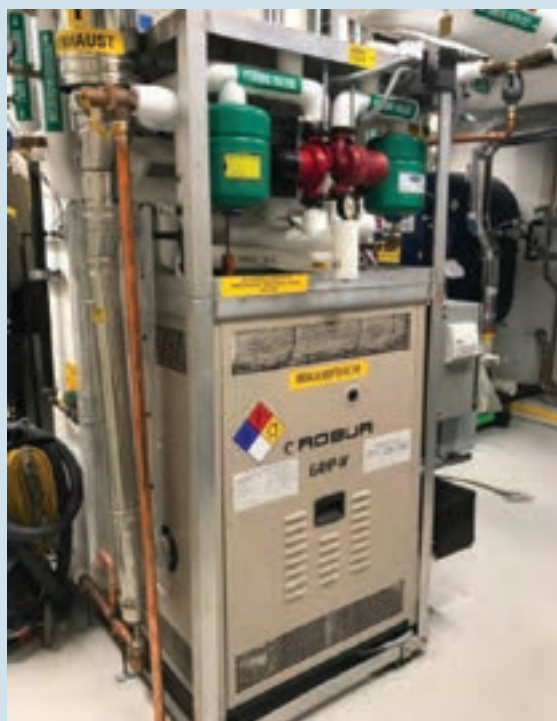
Wastewater Heat Recovery System at the Solaire in New York City (image courtesy of Natural Systems Utilities)
