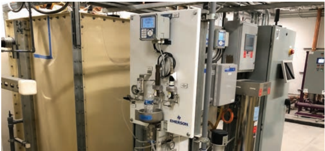
Onsite reuse system at Uber HQ (image courtesy of HTEC)
