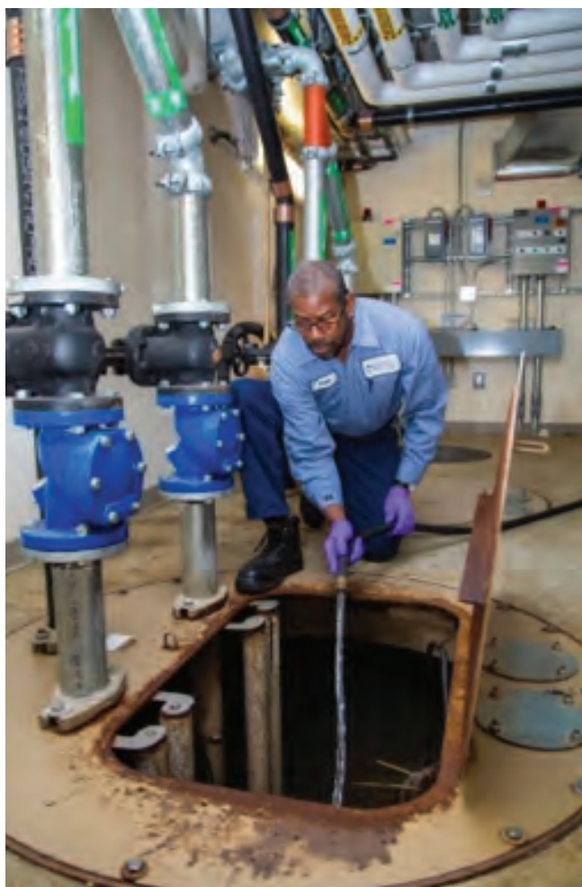
An Operator of an Onsite Water Treatment System
