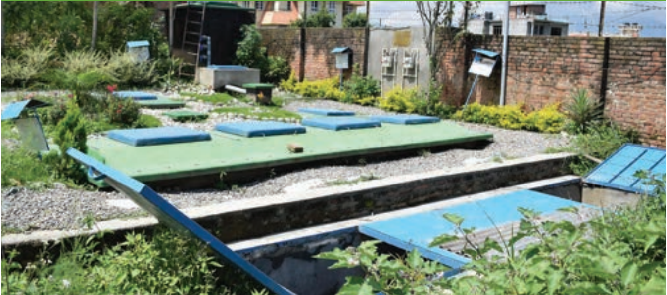
A view of the treatment plant's prefabricated modules (photo courtesy of ENPHO)
