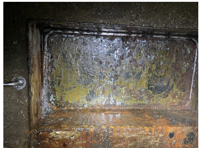
Brannan CSD Leaking Butterfly Valve.
