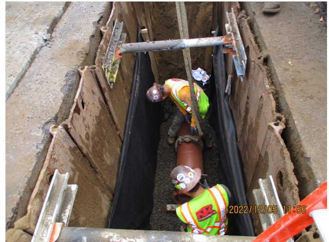
Segment B: South Side 12in VCP Installation at Ulloa St between 14th-15th Ave by NTK.
