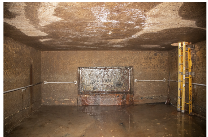
Leaky backflow preventor valve at Baker CSD.
