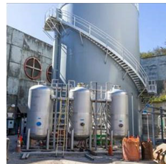
The Gas Holder Tank Building 741 digester gas piping and siloxane removal system.
