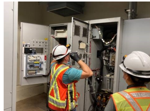
North Shore Site Visit: Dry Weather Pump Variable Frequency Drive (VFD)
