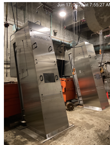
Completed bar screens in operation
