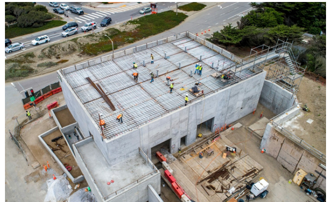
Contractor installing rebar reinforcement at new Electrical Building Roof as of September 2022.
