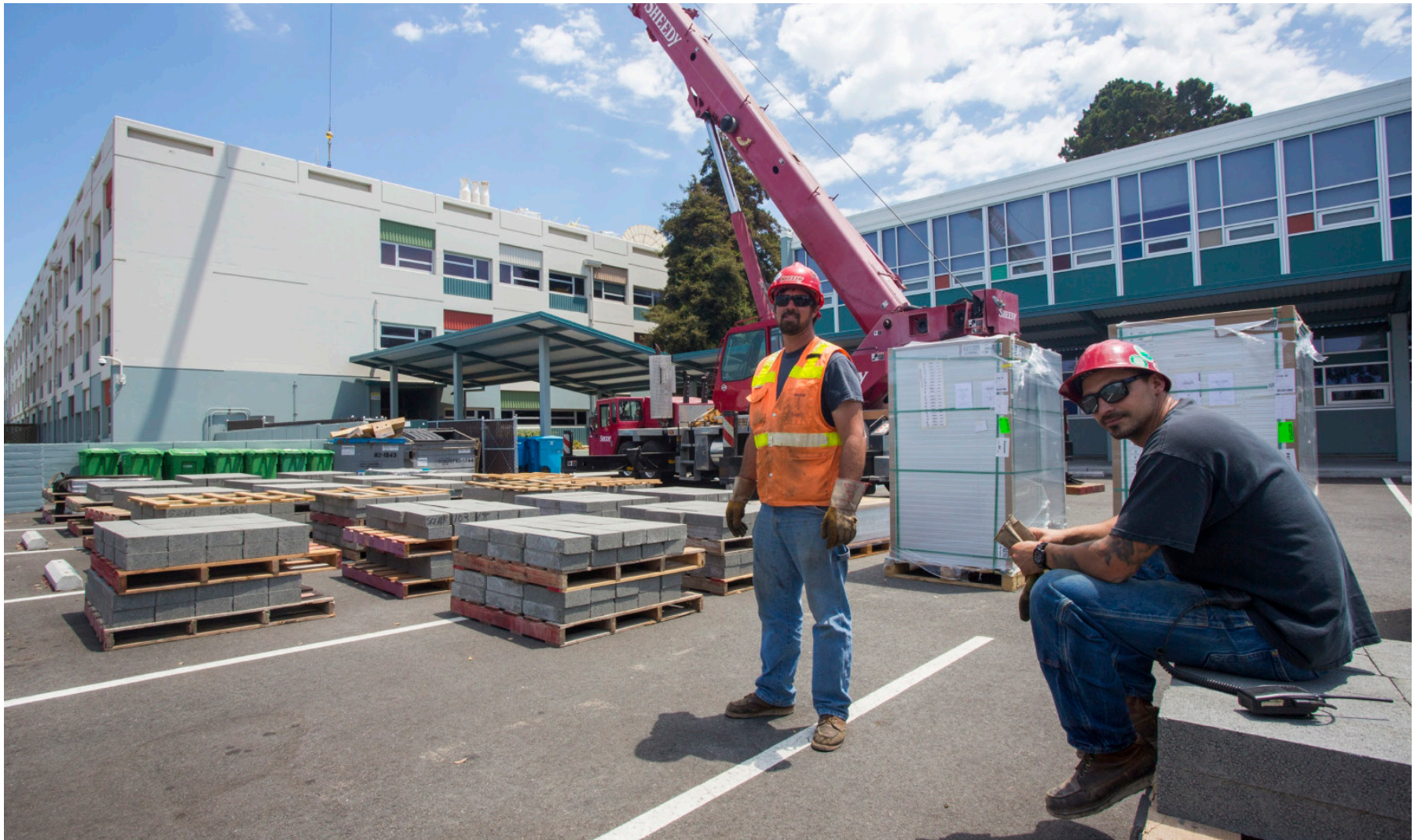
Burton High School solar installation
