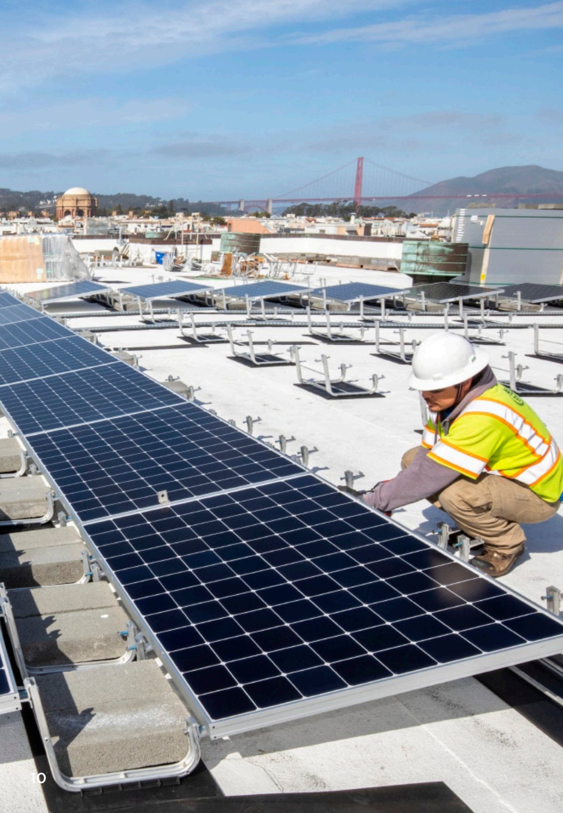
Solar panels installed at Marina Middle School
